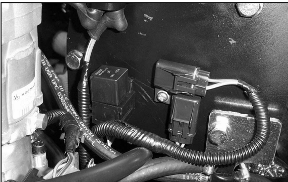
Located rear side of valve mounting bracket.
